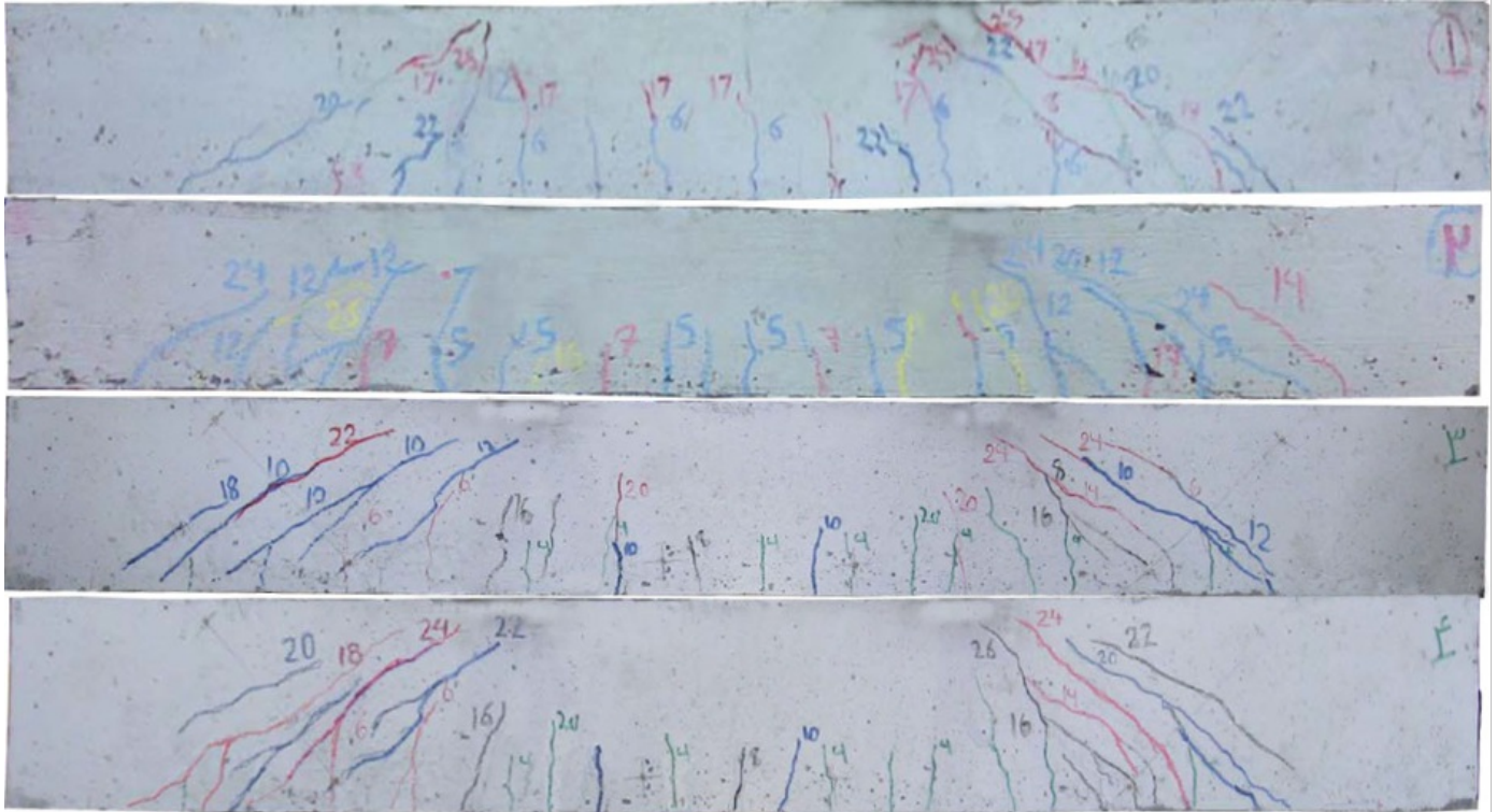
Figure 9. Appearance of cracks for the beams subjected to ultimate loads ( f_c=80 MPa)
