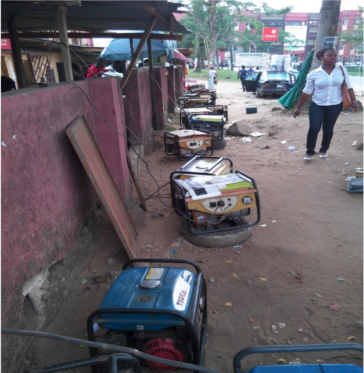
Plate 1. Generators as a major source of noise
